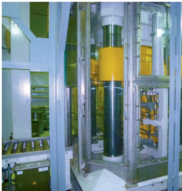
Figure 2. Super-compaction facility FSC004
